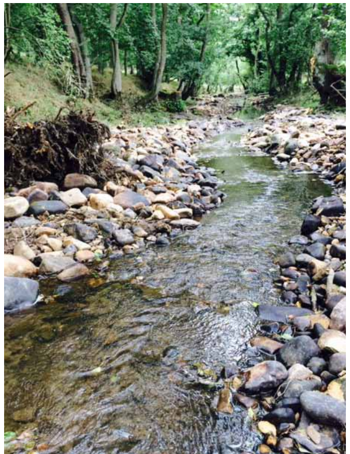
After works, the flow is concentrated into a deeper riffle-pool- run sequence
