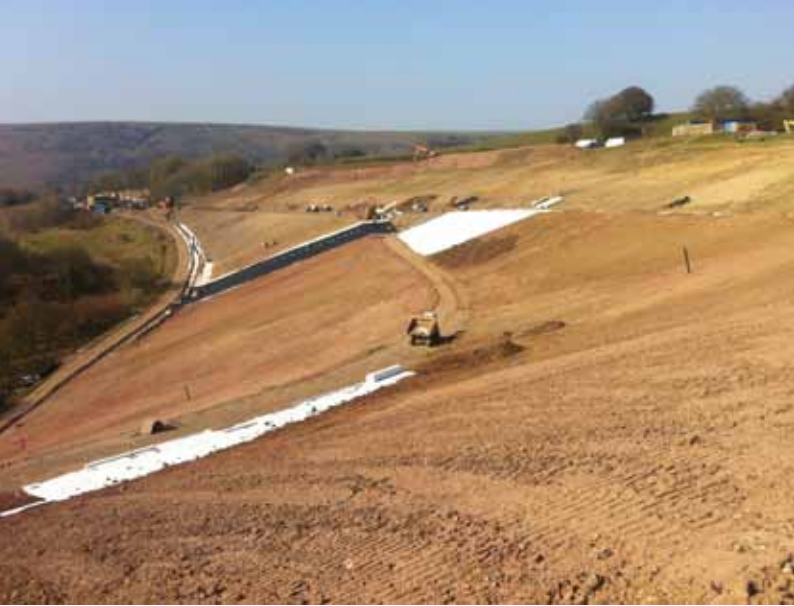
Erosion prone slopes in September 2015
