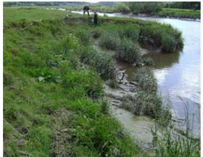
Large scour hole on the intertidal Tywi River threatens high pressure gas pipeline
