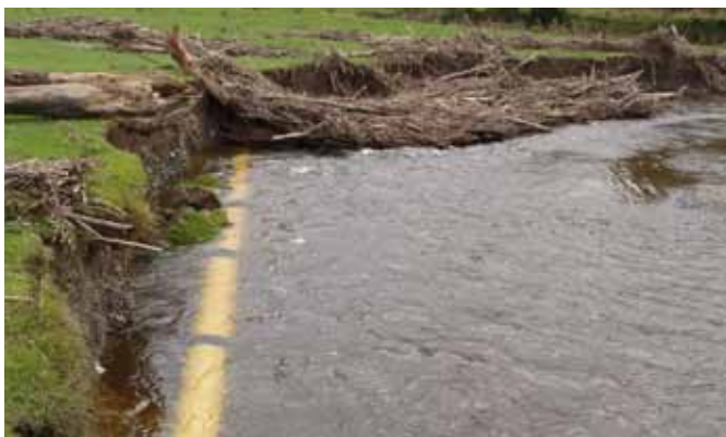
Over 30m of high pressure gas pipeline exposed by erosion
