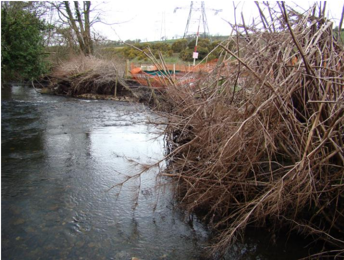
Eroded bank prior to works
