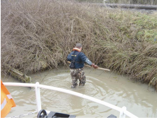
Surveying erosion and failed piling
