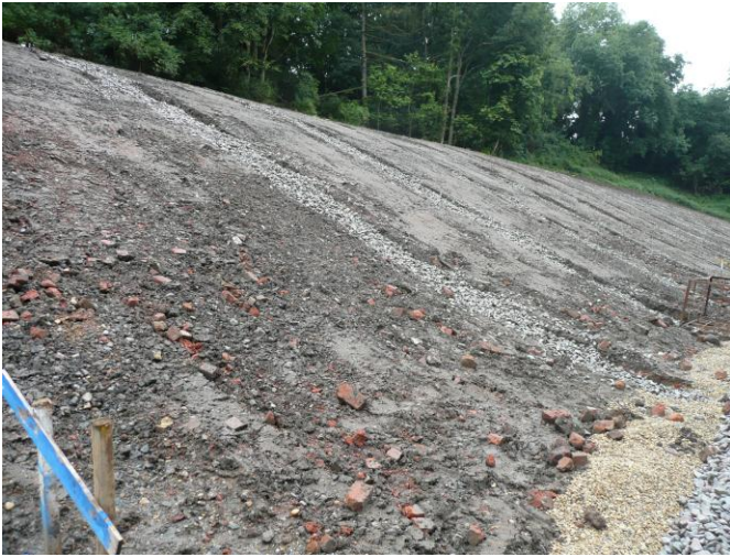
Poor underlying ground conditions
