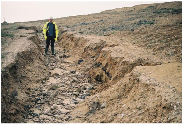
48hr flood event created severe scour
